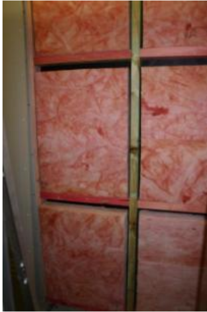
Figure 21: R 2.8 glasswool insulation fitted with 3% gaps at side and 6% gap at the top of each frame cavity (D4862b)
