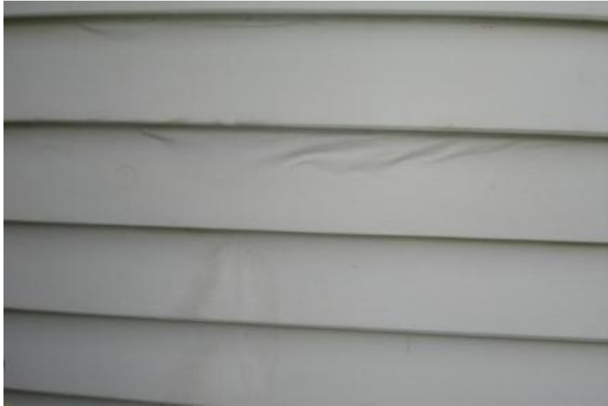
Figure 12: Blistering paint on weatherboard, evident after Airfoam installation (House W3)
