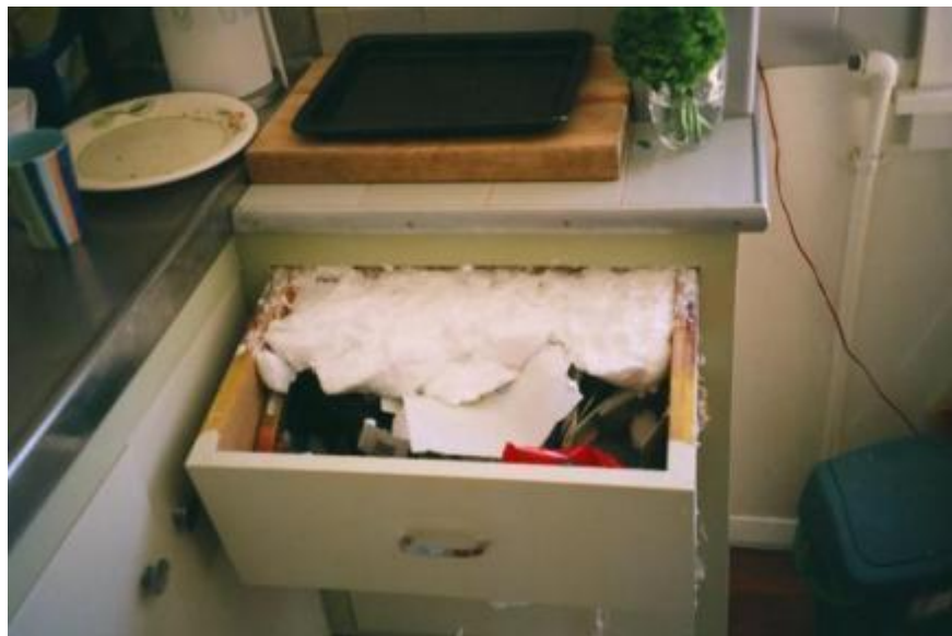
Figure 1: Example of serious installation problems (House W7)
