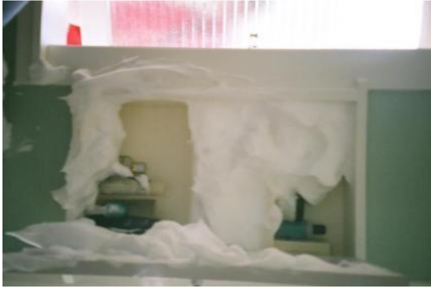
Figure 2: Example of serious installation problems (House W7)
