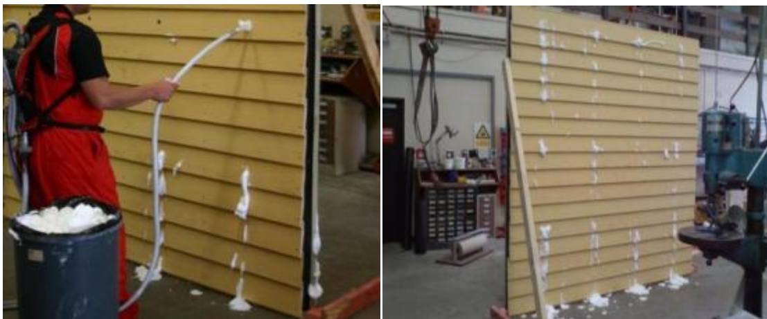
Figure 13a & b: Installation of Airfoam in large scale test wall (D4861) at BRANZ
