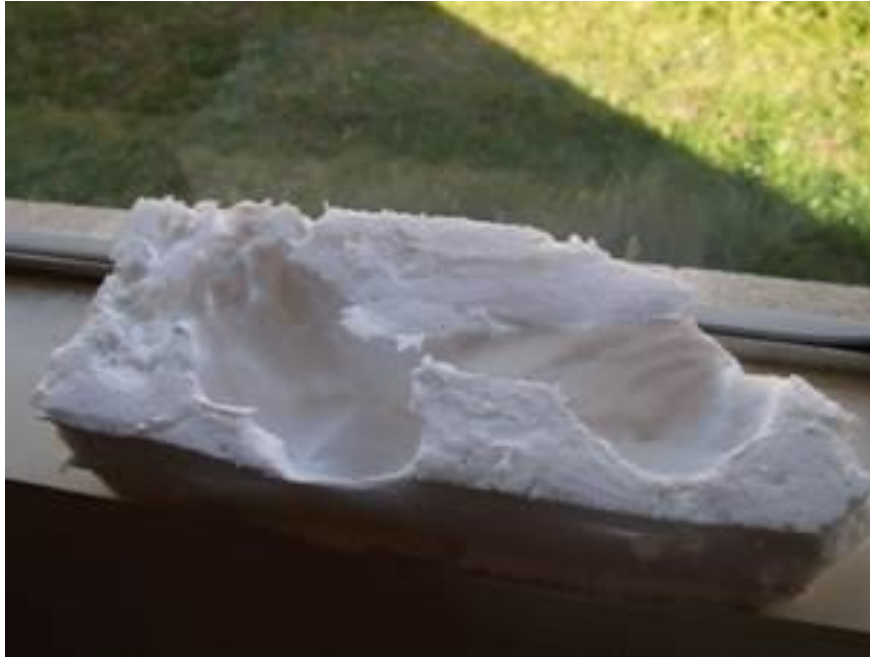
Figure 9: Airfoam sample removed from wall cavity showing voids (House W4)
