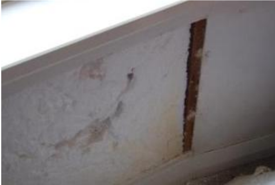
Figure 10: Removal of wallboard to assess Airfoam installation – note voids present house (House W3)
