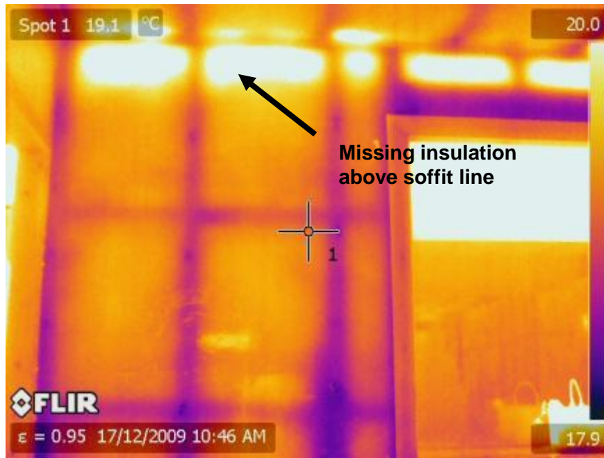
Figure 4: Thermal image identifying missing insulation in another upper wall above the soffit line (House C7)
