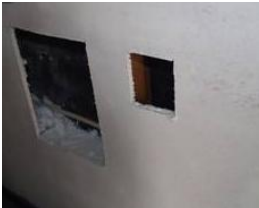
Figure 8: Removal of wallboard confirms missing insulation (House W4)
